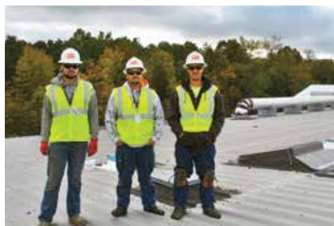
Noah Hoepfner, Daniel Turner and Daniel Baker, working for CEI Group, LLC, apply sealer coating on the roof of Aero Auto.
